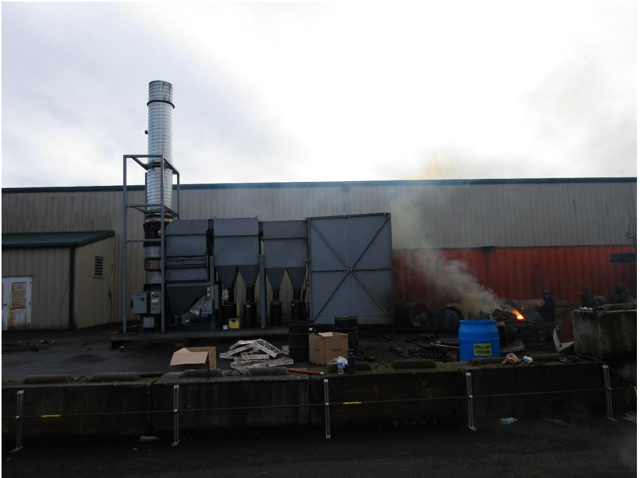
Multi-Clone / HEPA Filter System – January 30, 2020
