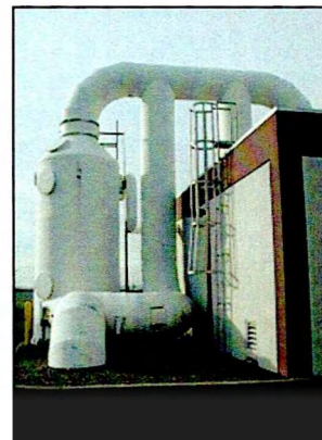
Fig. 3: The odor control scrubber.
