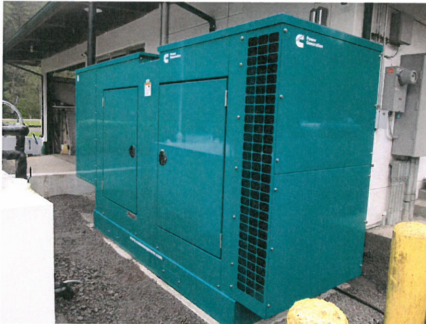
Washougal Hatchery Buildings Emergency Generator – April 23, 2015
