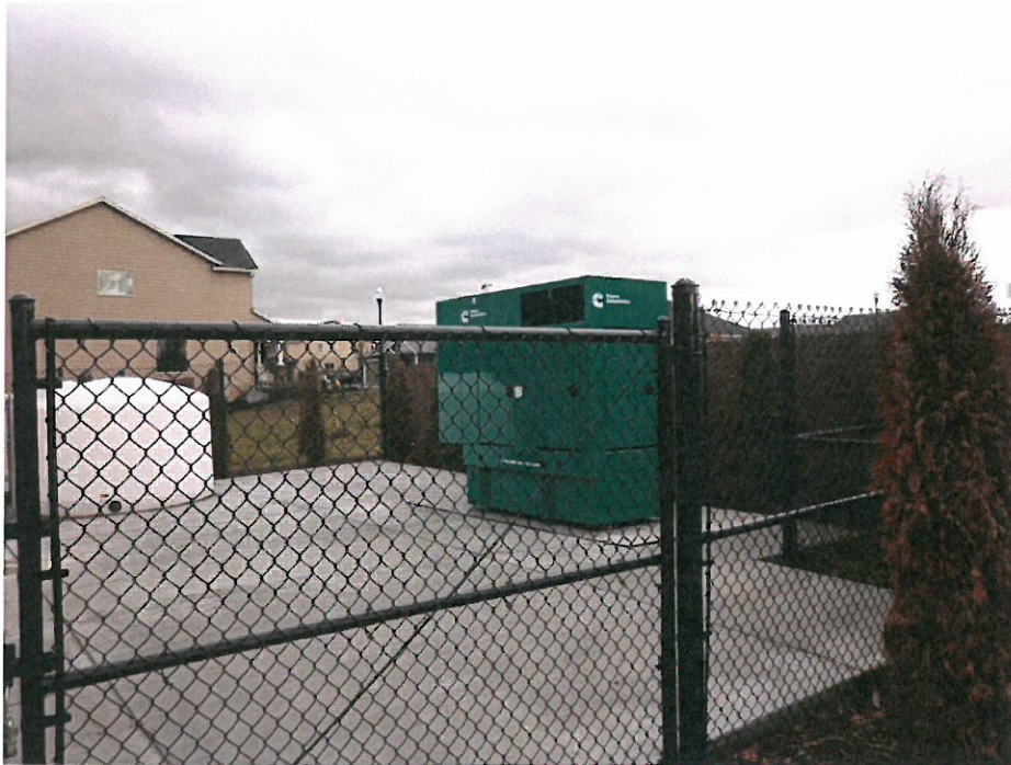
Dunning Meadows Wastewater Pump Station Emergency Generator Engine November 25, 2014
