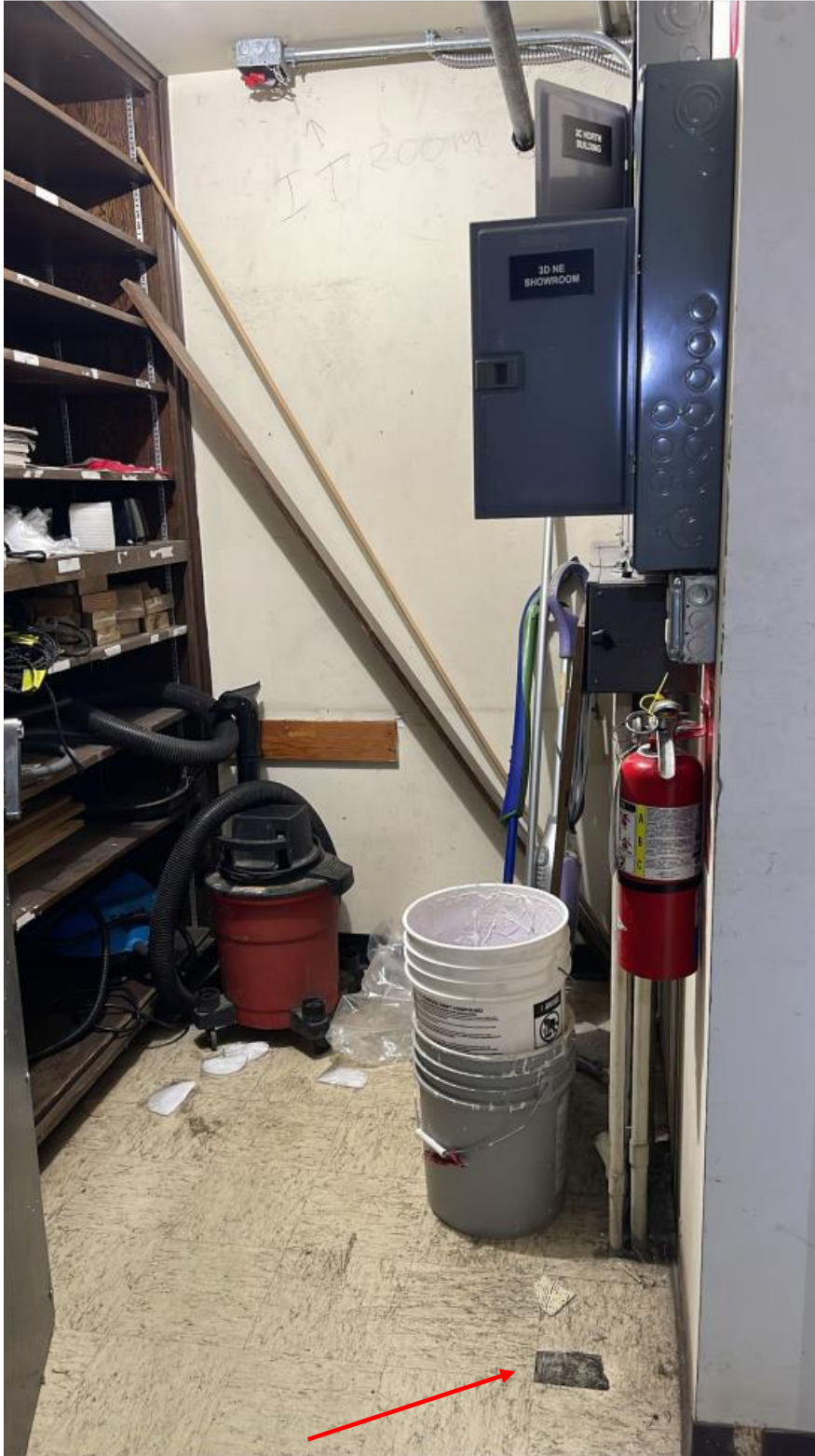
Storage closet ACM floor tiles & mastic.
